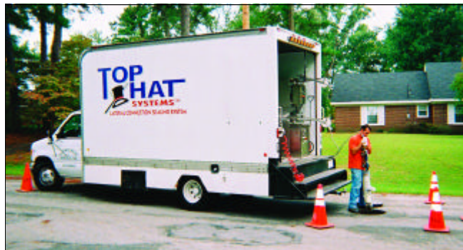
Southwest Pipeline and Trenchless Corp. Top Hat crew placing Top Hat applicator into manhole.
